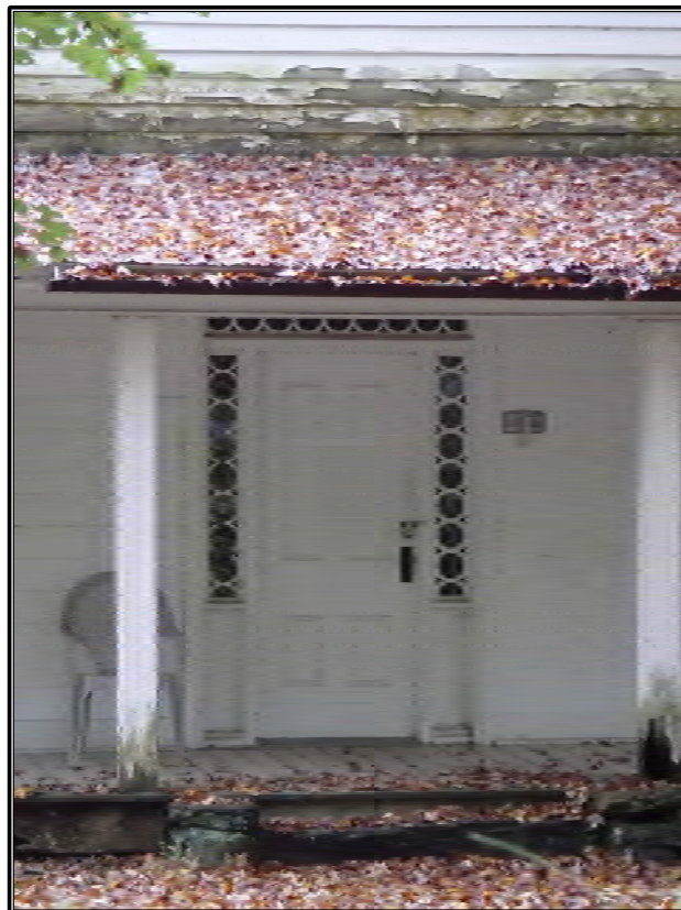
Figure 27. Detail of entry of the Frank Seagraves House (AH 191), at 1538 Little Helton Road with similar trim on sidelights and transom, facing south.
